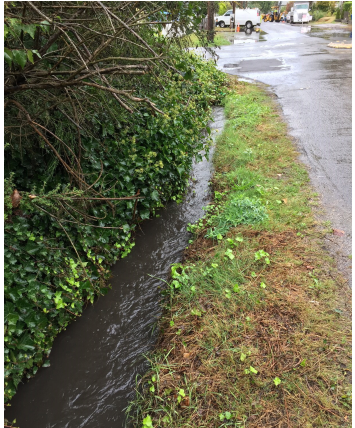
Figure A ditch on NW 17th Street running high - because this segment receives high flows from upstream and is relatively flat, it tends to clog.
