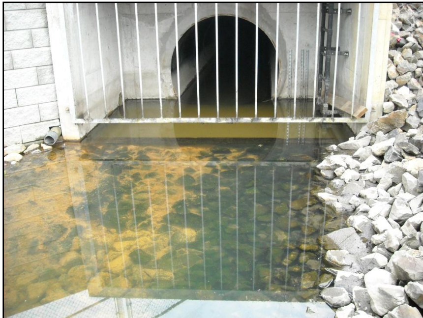
Figure 2.2.2.3c. Photograph of I1 Diversion Structure and Outfall
