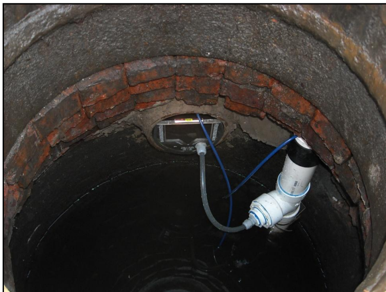
Figure 4.2.2.1a. Photo of Thel-Mar Weir in Downstream Outlet Pipe of CBSF2
