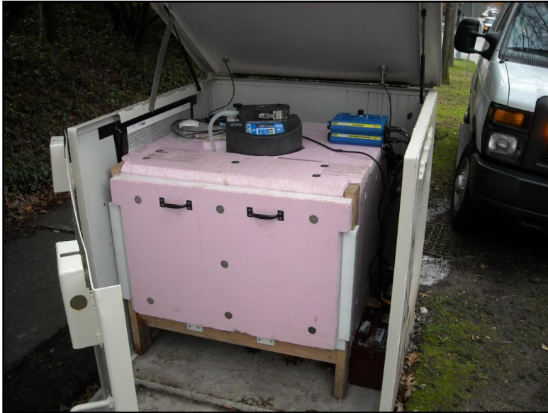
Figure 2.2.2.b. Photograph of C1 Equipment Cabinet
