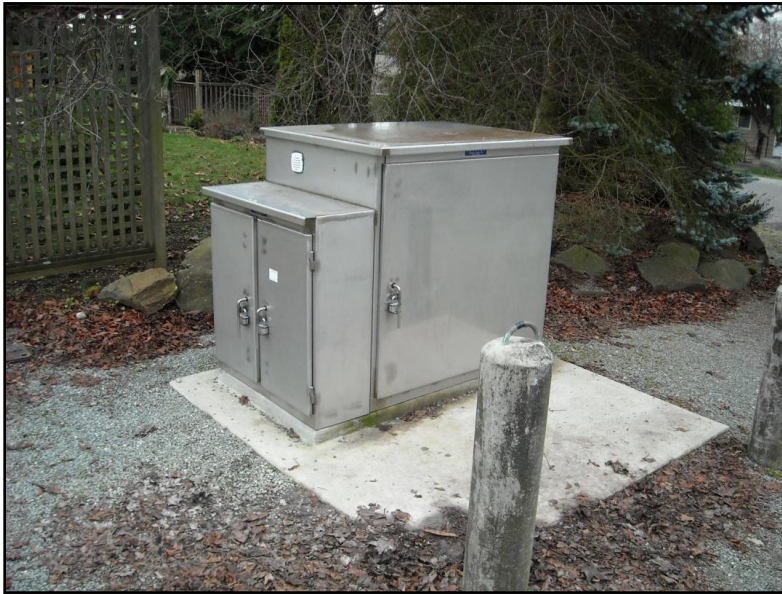
Figure 2.2.2.1c. Photo of R1 Equipment Cabinet
