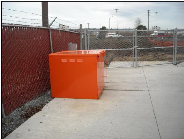
Figure 2.2.2.3d. Photograph of I1 Equipment Cabinet
