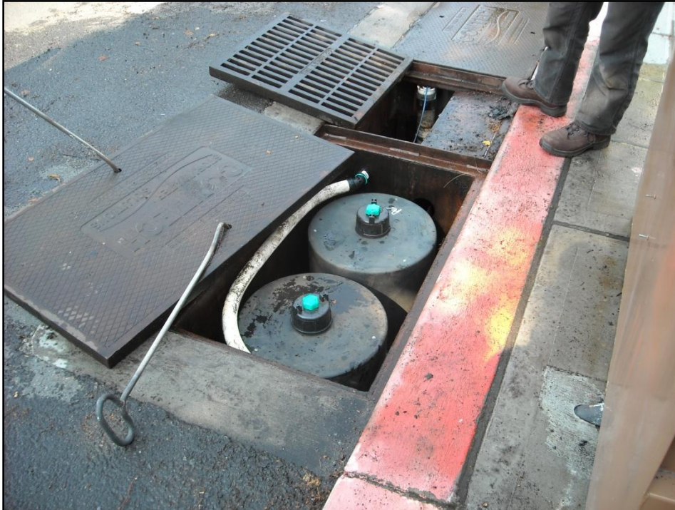
Figure 4.2.1e. Photo of CBSF1 with Covers Removed
