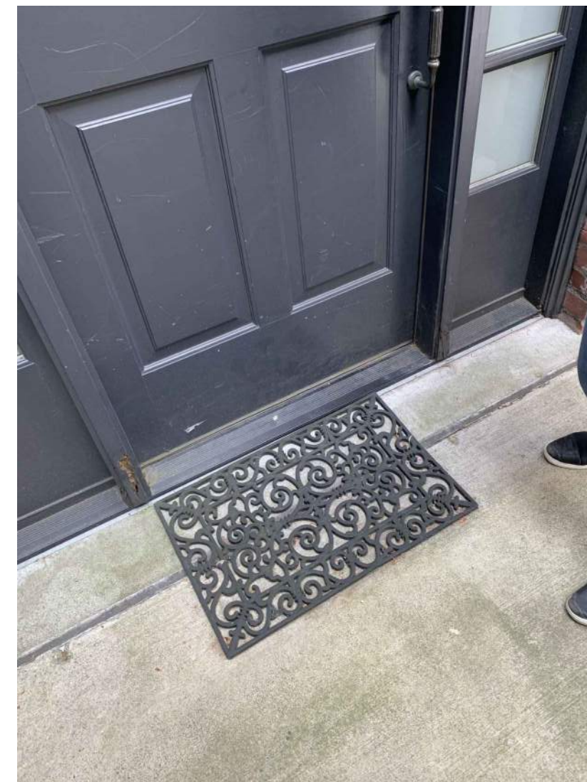
5 EXTERIOR FRAME DAMAGE EXAMPLE
