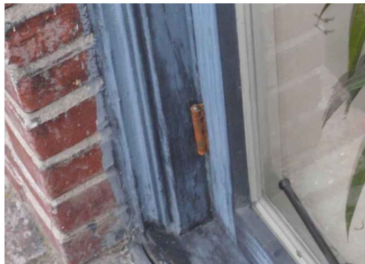
8 RUSTING WINDOW/DOOR HARDWARE EXAMPLE
