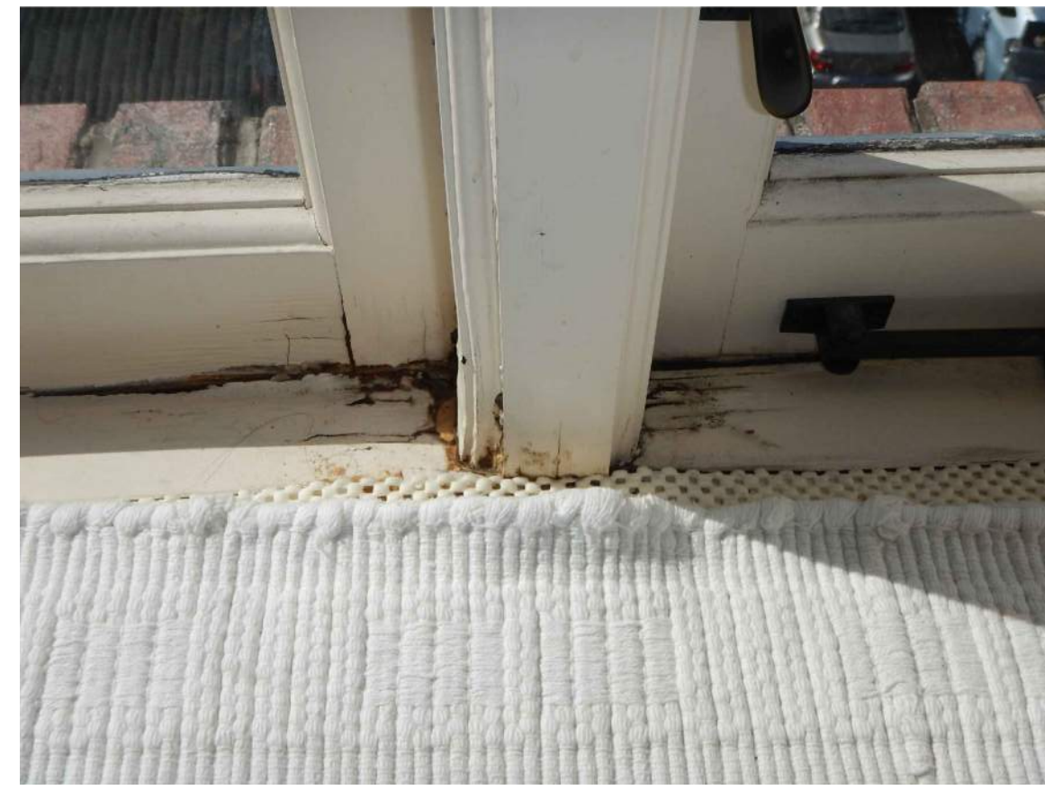
4 INTERIOR FRAME DAMAGE EXAMPLE
