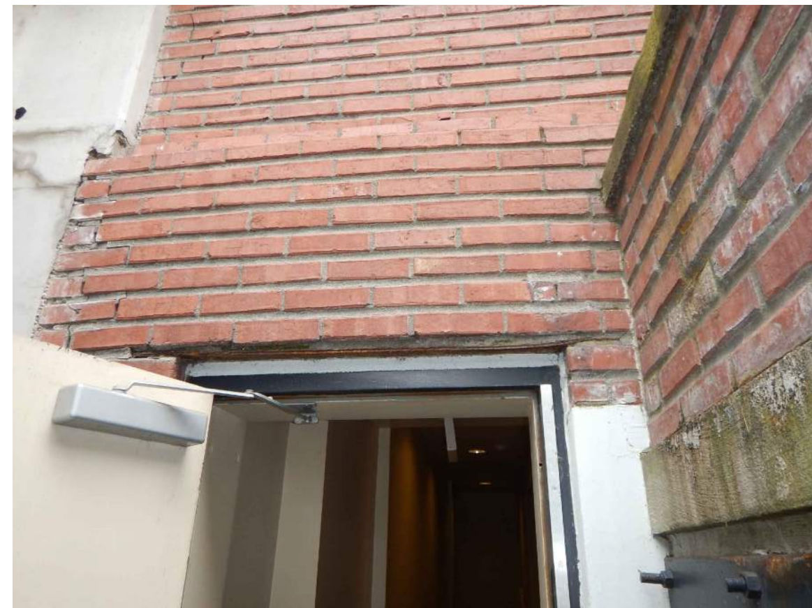
11 TYPICAL STEEL LINTEL IDENTIFIED FOR REPLACEMENT
