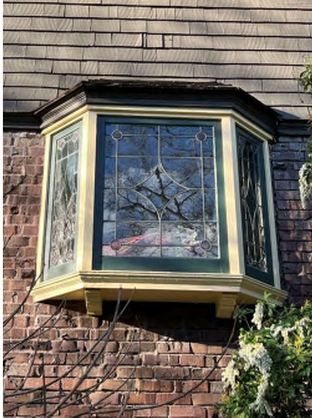
Figure 23. Oriel on the south side of the house, with three curved diamond leaded glass windows, supported by two corbels. (Author photo)
