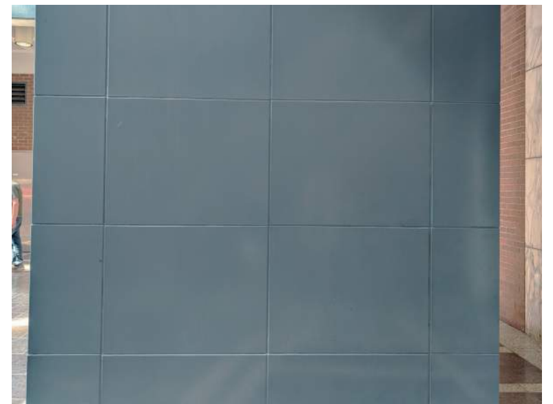
Existing "Pioneer Blue" Paint Color (Interior) New work to be painted to match
